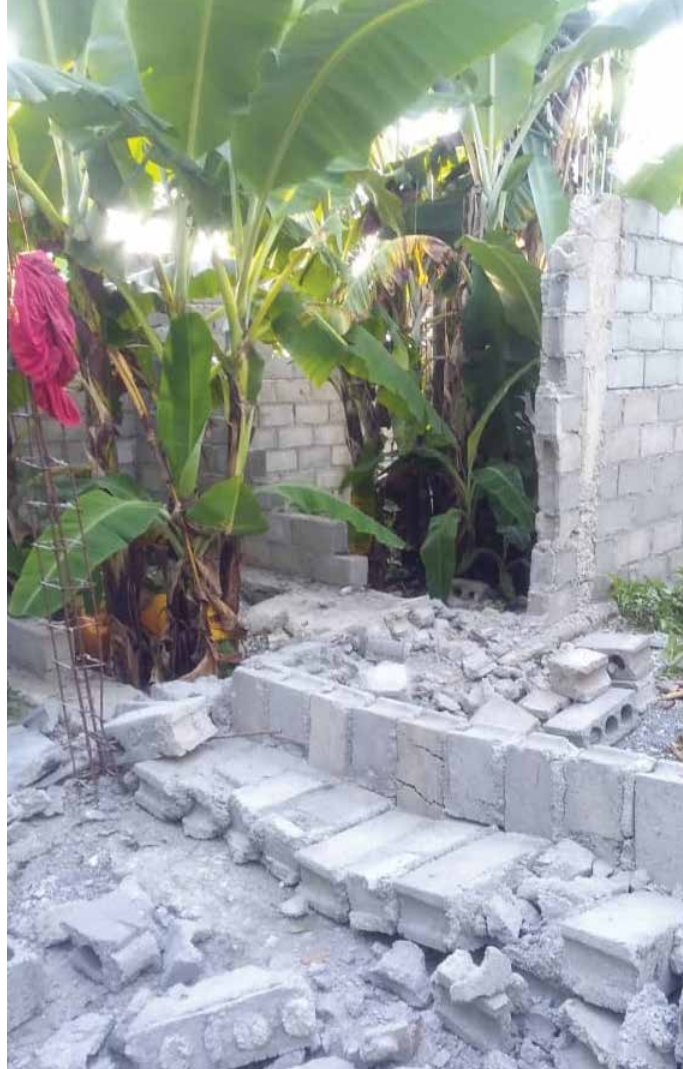
The Aug. 14, 2021, earthquake caused widespread damage to structures in the southwest part of Haiti.
